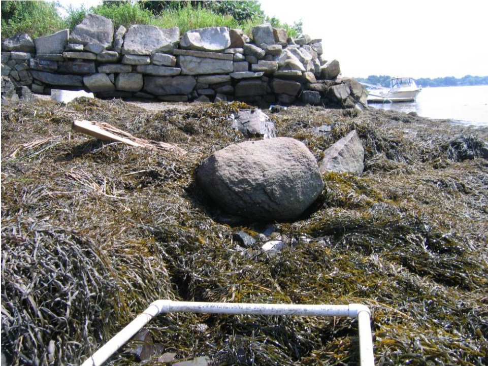
Figure 2 Cedar Point boat launch A) facing south B) facing north with boat launch and retaining wall.
